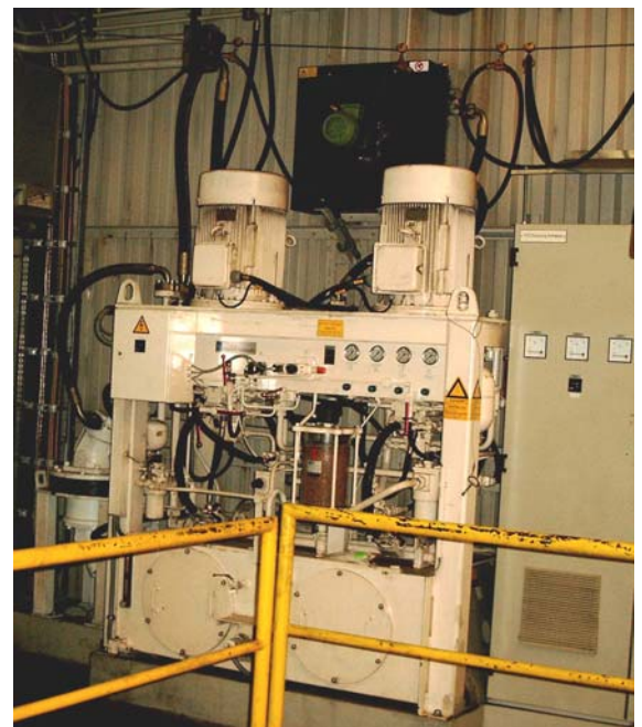
Fig. 26: Weather-protected and maintenance-friendly: Arrangement in the protective housing The photograph shows the oil cooler above the power pack in the wall of the protective housing
